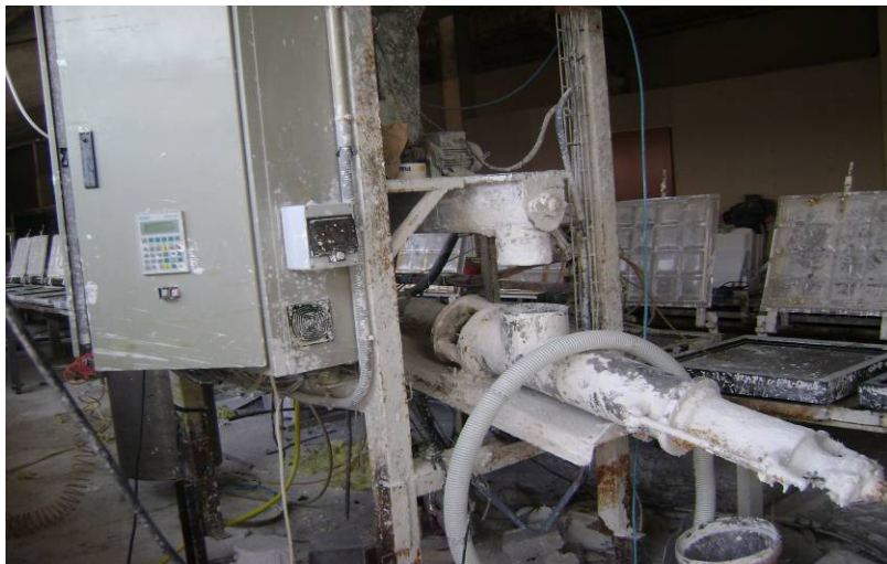
Fig.1. The kneader installation type "COROS OP5" SIEMENS [4].
