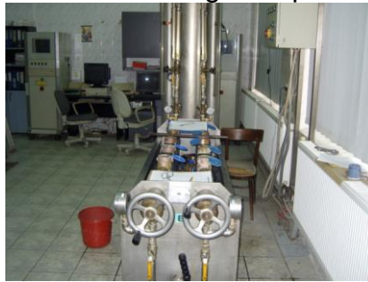
Figure 1. Metrological stand of water meters [1]
